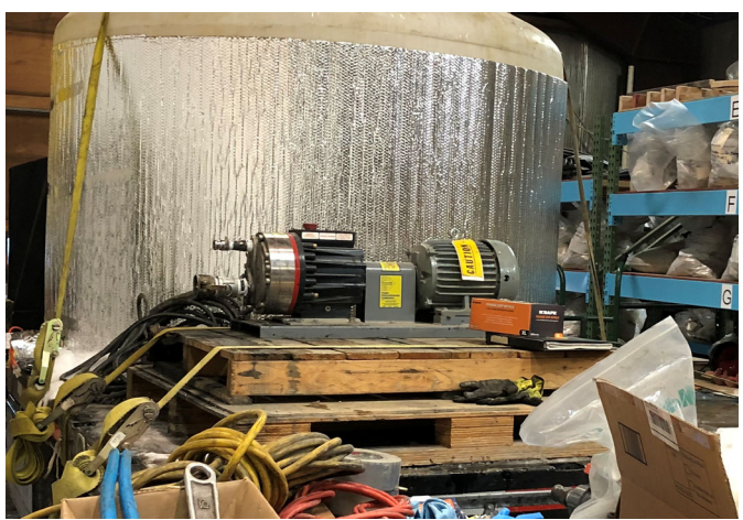
Photo 6: Injection pump 4, Hydracel pump. November 8, 2019
