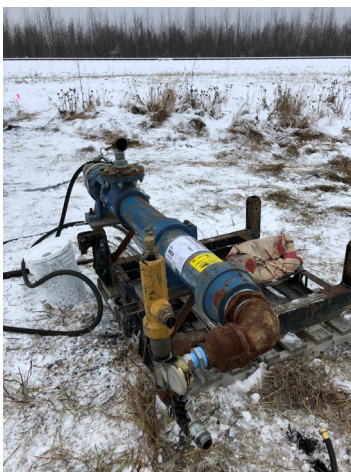
Photo 5: Injection pump 3, GeoTek pump. November 2, 2019
