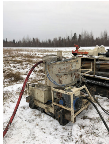
Photo 4: Injection pump 2, Moyno Pump. November 1, 2019
