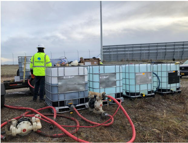
Photo 3: Injection Pump 1, diaphragm pump. October 29, 2019
